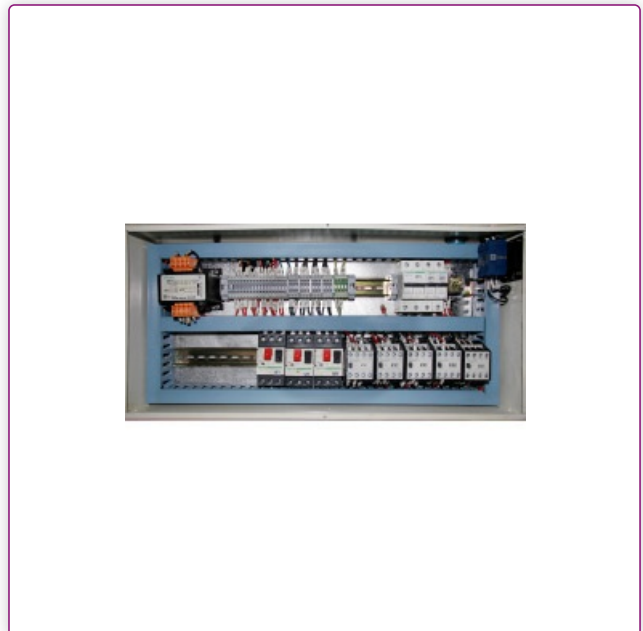
DC control cabinet
