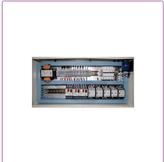
DC control cabinet
